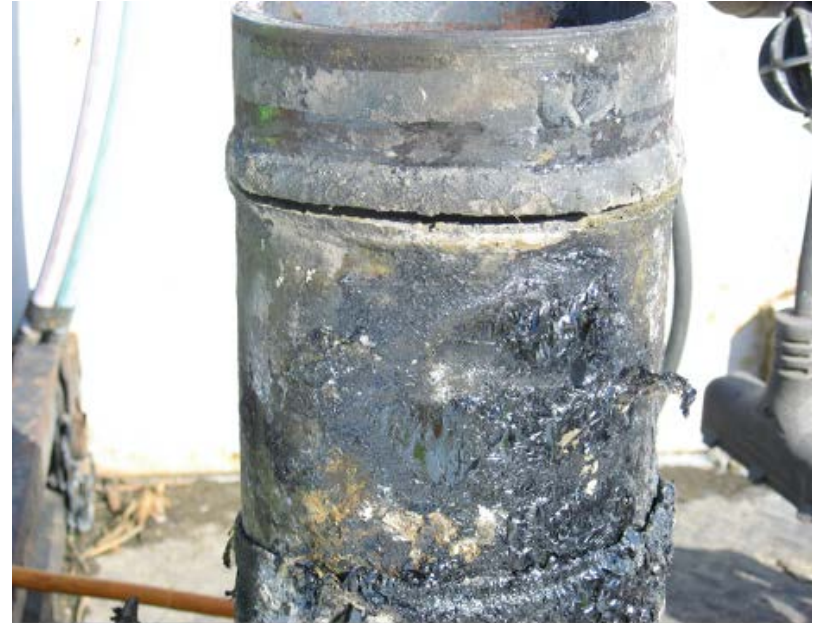
UM-Crookston Ruptured Natural Gas Main
